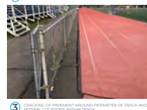
3 CRACKING OF PAVEMENT AROUND PERIMETER OF TRACK AND SEVERAL LOCATIONS WITHIN TRACK
