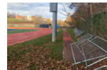
5 POLE VAULT RUNWAY HAS STRUCTURAL ISSUES. LANDING AREA VIEW SUDE TO TRAMPOLINE
